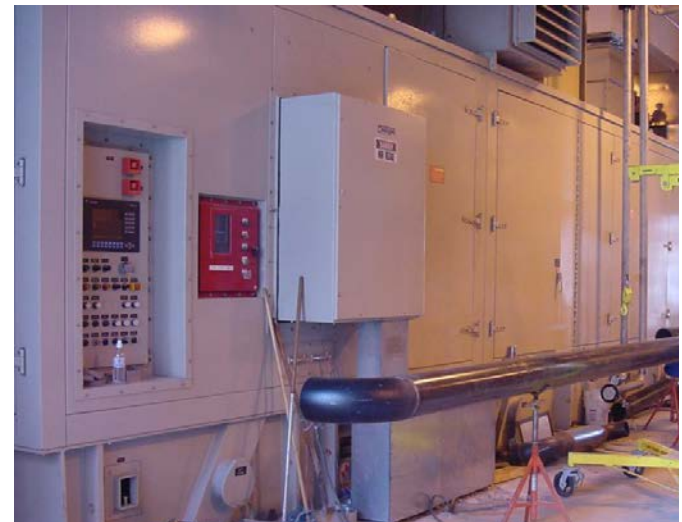
7.0 MW Solar Taurus Turbine Generator
