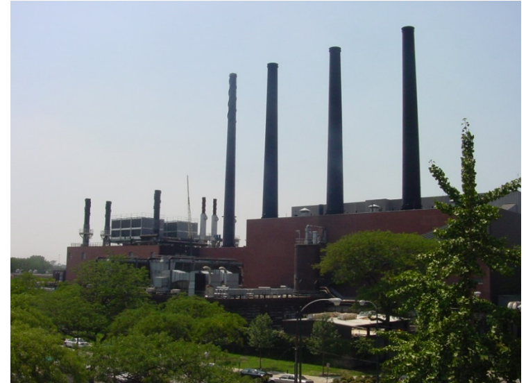
UIC West Campus CHP Facility
