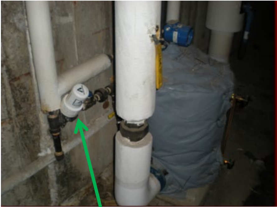
Steam Trap & Remote Monitoring Device
